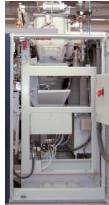
Air entrainment system
