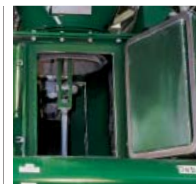
Pressure chamber with maintenance door
