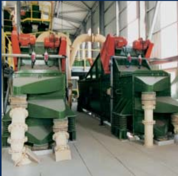
HAYER sand processing plant
