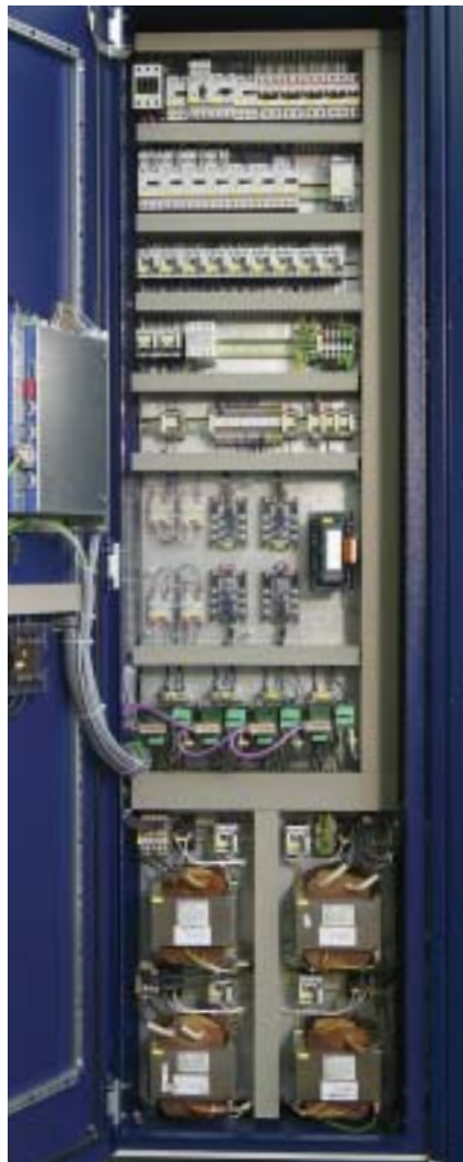
Control panels integrated in the machine enclosure power element
